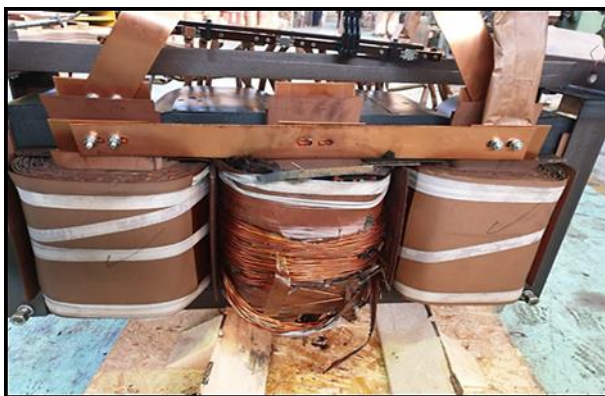
Figure 2. Destroyed windings after short circuit current
