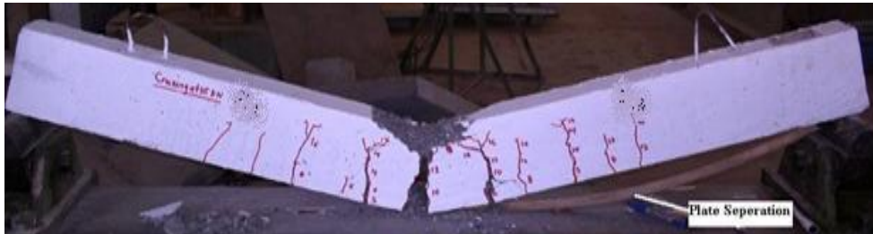
Fig .(6) Failure Mode by Separating Steel Plate
