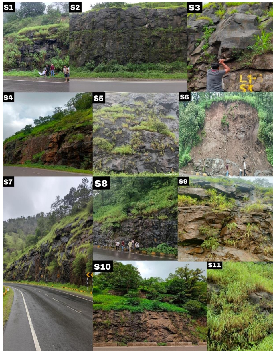
Figure 4. Field photographs depicting the condition of investigated slopes along NH3 (S1, S2, etc. Names of Slopes for field identification).
