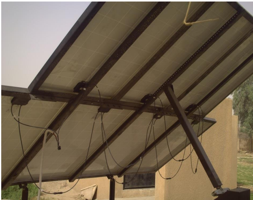
Fig. 10 An image shows the Installation platform for solar panels.
