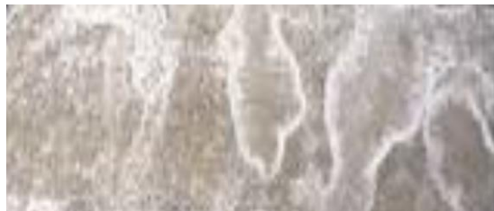
Figure 16. The effect of groundwater salinity on the concrete surface.
