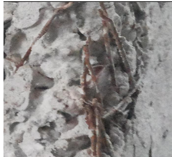
Figure 18. The effect of concrete corrosion on steel fiber located near the surface of the concrete beam.
