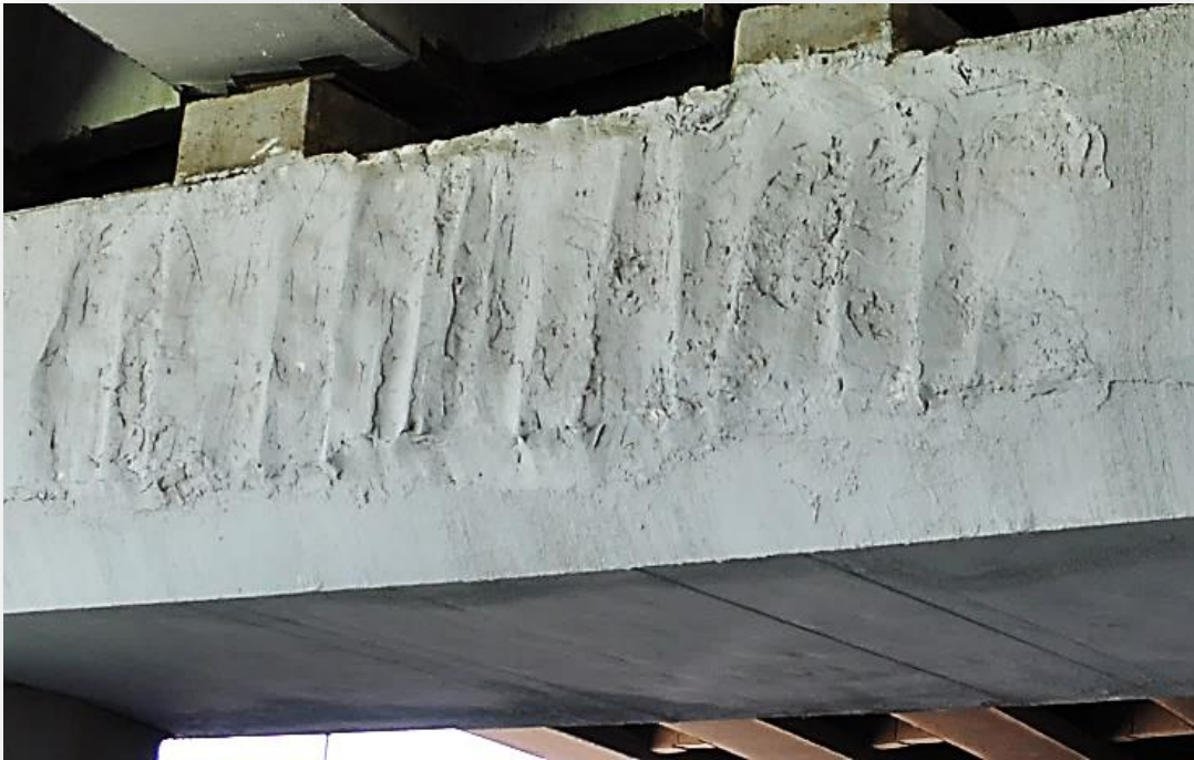
Fig. 15 Poorly repaired area in pier capital (just by plastering).
