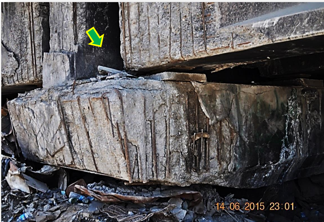
Fig. 13 The disappearance of the concrete cover and exposure of reinforcement of pier capital and girders.
