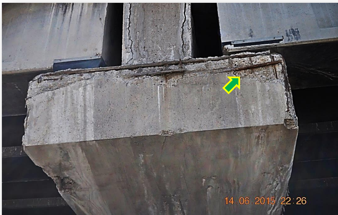
Fig. 6 Cracks, Delamination and Reinforcement exposure of Pier Capital due to heavy traffic & low strength of concrete cover.
