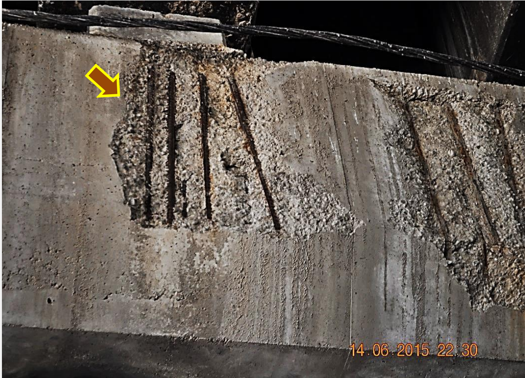
Fig. 9 Spalling and exposure of reinforcement in pier capital due to heavy traffic loads and low concrete strength.
