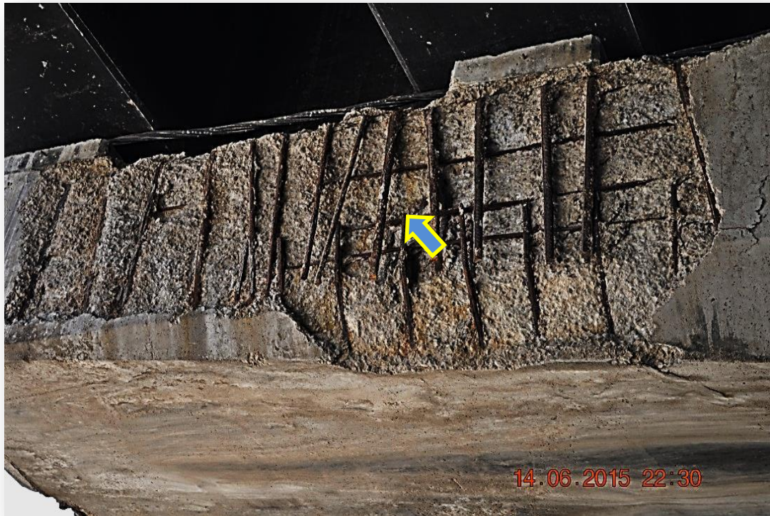
Fig. 5 Concrete delamination and exposure of Reinforcement in pier Capital due to heavy traffic loads & low strength of concrete cover.
