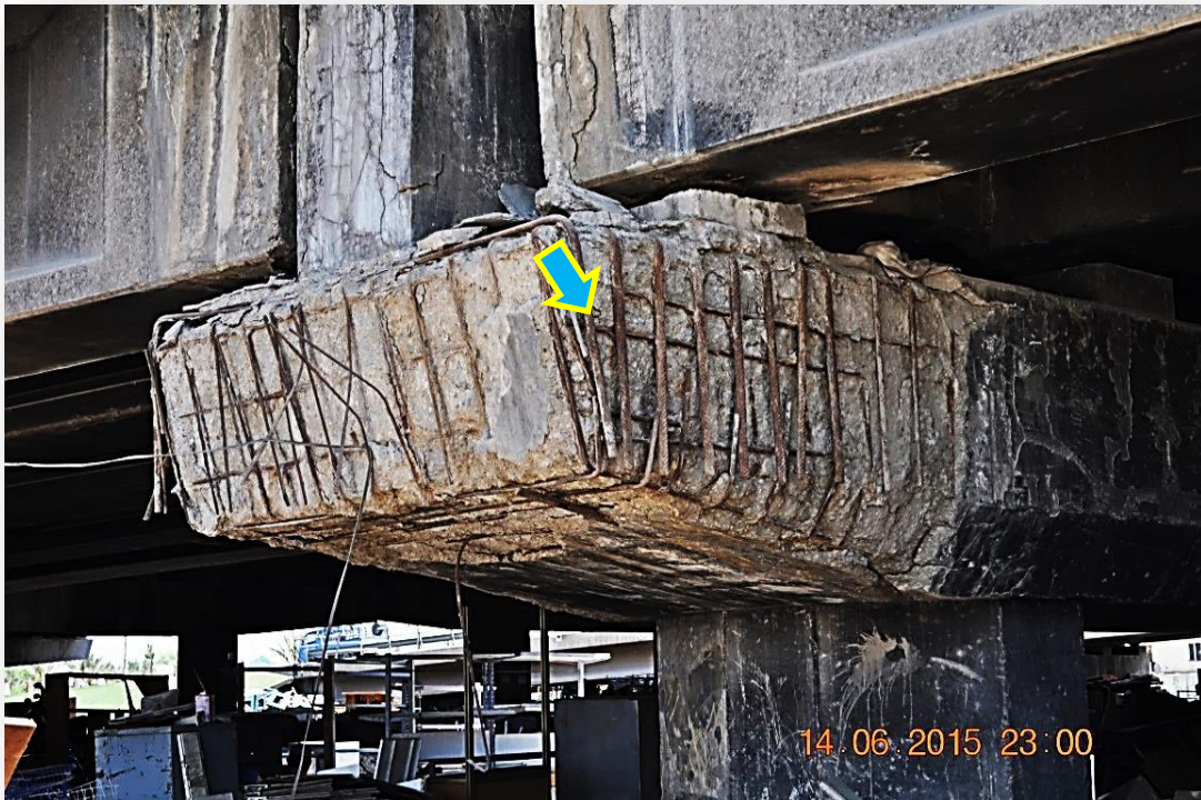
Fig. 12 The disappearance of the concrete cover and exposure of reinforcement of pier capital due to heavy loads & badly constructed.
