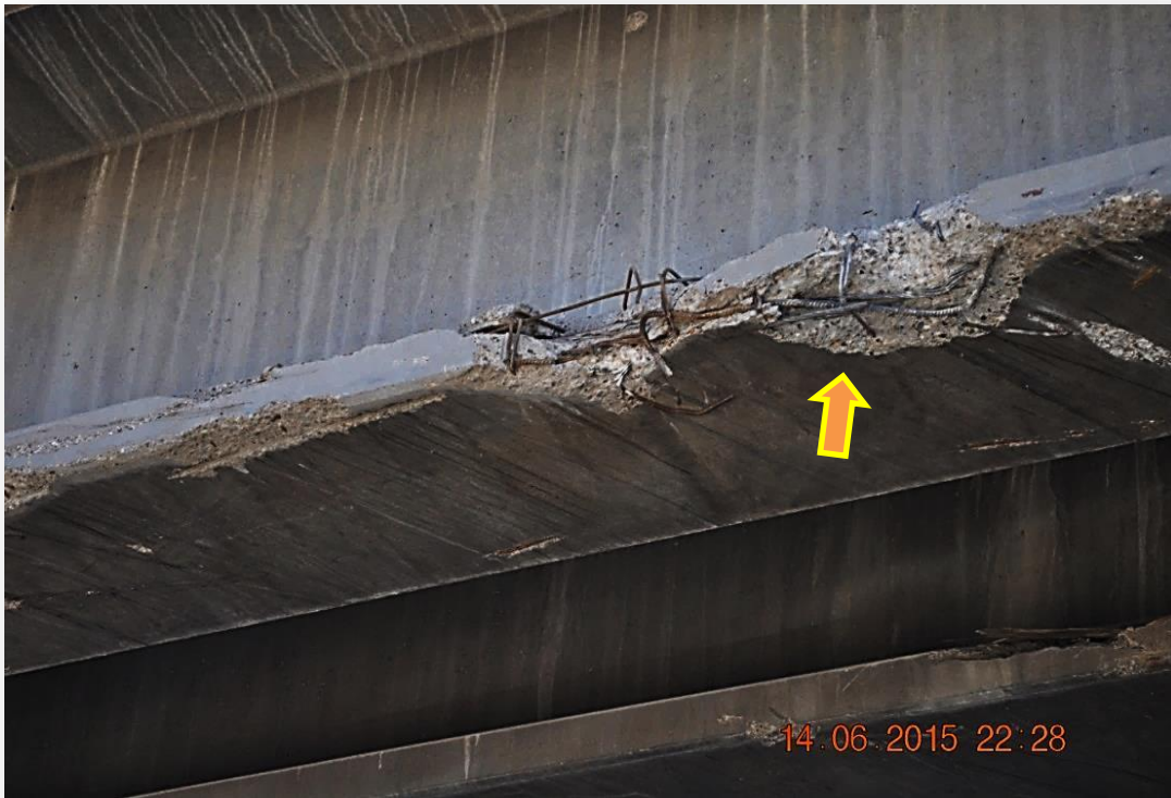
Fig. 7 Cut in wires of the girder flange due to crash with high-rise vehicles.
