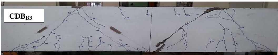
Figure 11. Crack pattern for beam CDB B3 after testing
