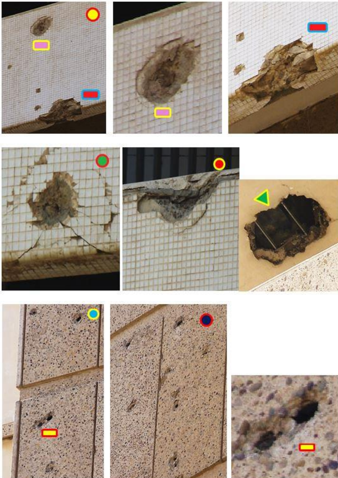
Fig. 9 Damages caused by projectiles at an estimated height of 25-45m (Pentax K-x with MTO 1100mm 10.5).
