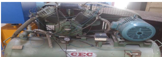
Figure:4 Photographic view of two-stage reciprocating compressor
