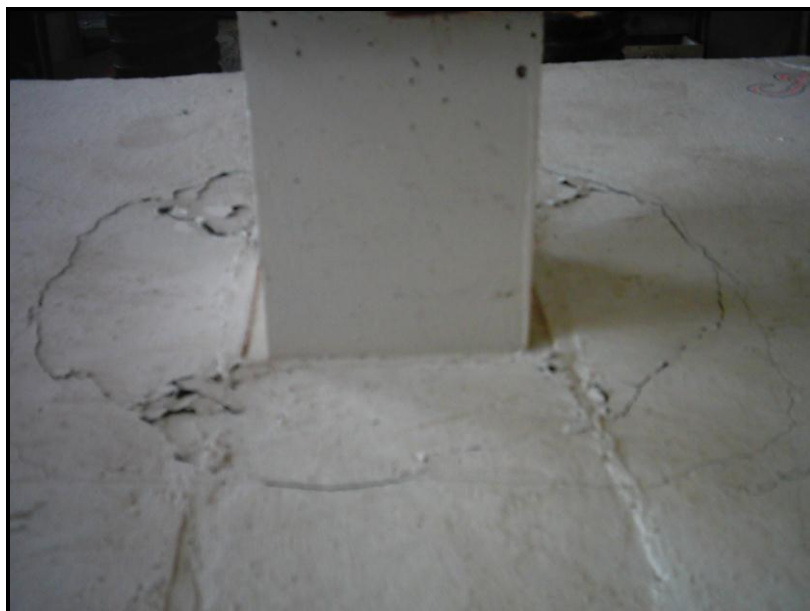
Figure (5) Compression surface of tested slabs after failure
