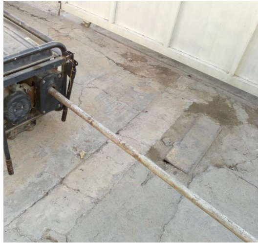
Figure 5: 6 meter exhaust pipe
