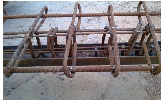
Plate 4-b: The steel reinforcing bar cage resting on the steel channel (with welded headed studs) for a typical test beam.
